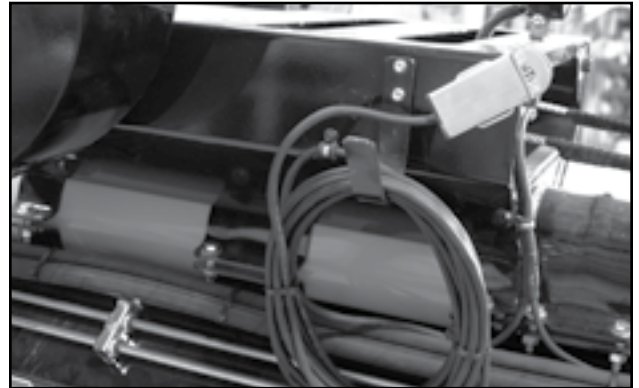
Fig 34 - Conveyor belt control switch
